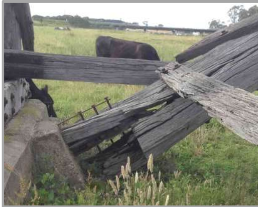
Nicholson River bridge: Base of the south east bracing stay, with cattle grazing nearby, Princes Highway in the background
