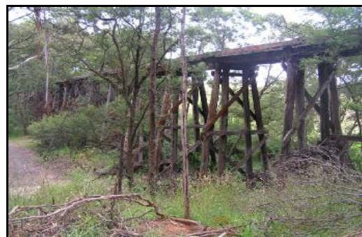
As it was before being completely destroyed by the fire.
